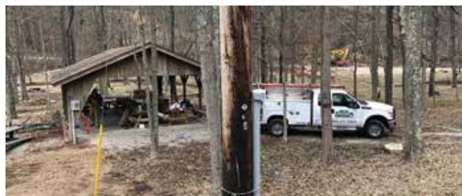
HARD AT WORK: REA Energy Services employees install electricity to Blackleggs Memorial Park.
